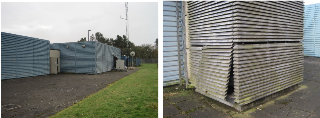
Figure 4 Bathgate Control Building
